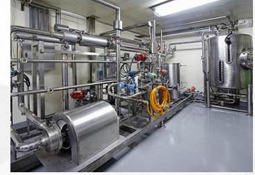
Membrane Filtration System
