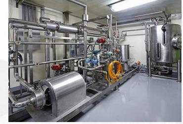
Membrane Filtration System
