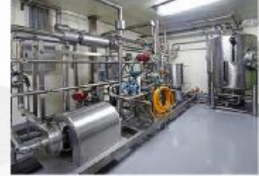
Membrane Filtration System
