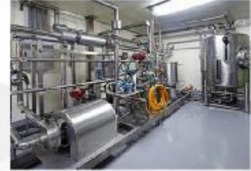
Membrane Filtration System
